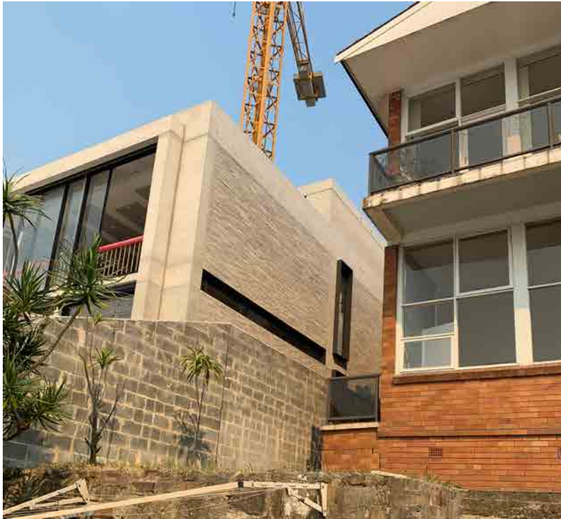
View south-west of the interface with 3 Bay View Street showing extensive boundary walls and northern windows.
