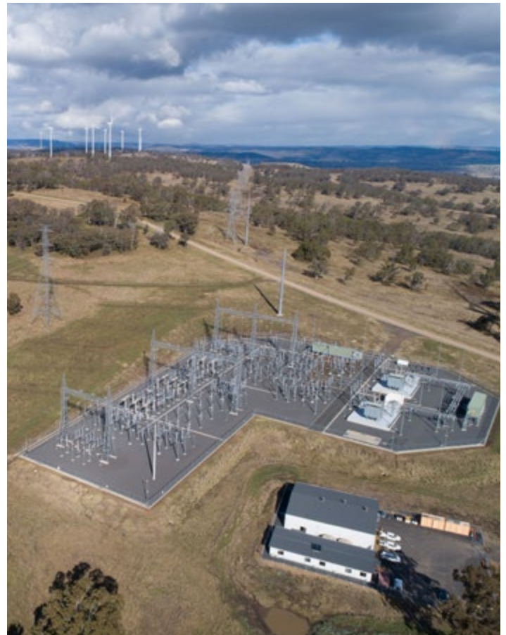
Renewable energy infrastructure, Inverell
