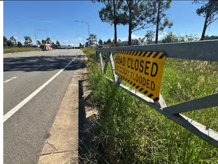
Photograph 08. Grange Avenue Flood Gate (Bells Creek Crossing)
