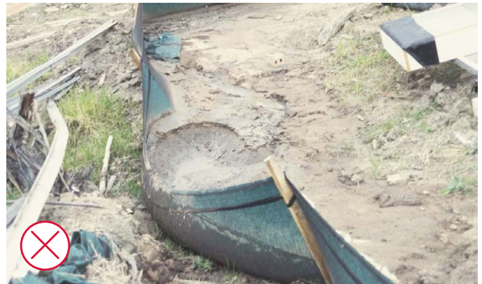
A poor example of a sediment fence that has been inappropriately managed. Source: Catchments and Creeks Pty Ltd.
