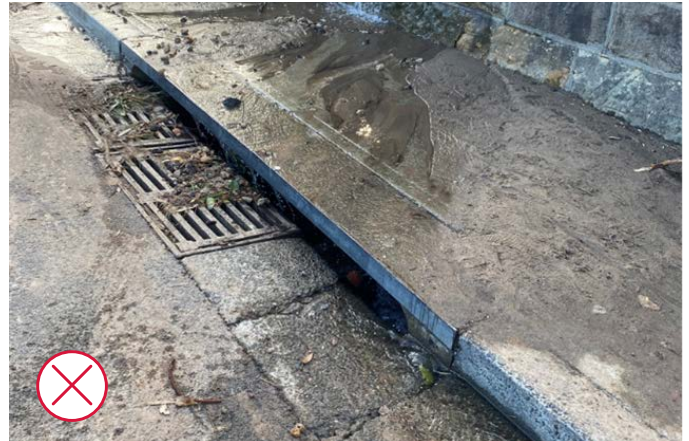
A poor example of gutter protection as sediment enters a stormwater drain.
